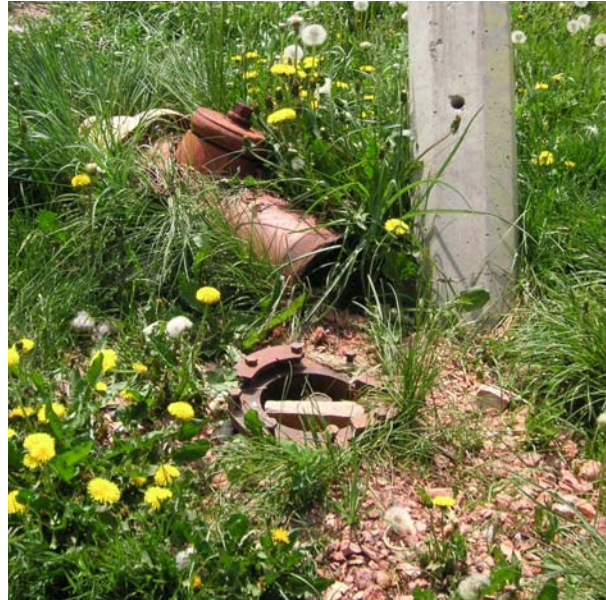
Inoperable hydrant at Muddy Creek
