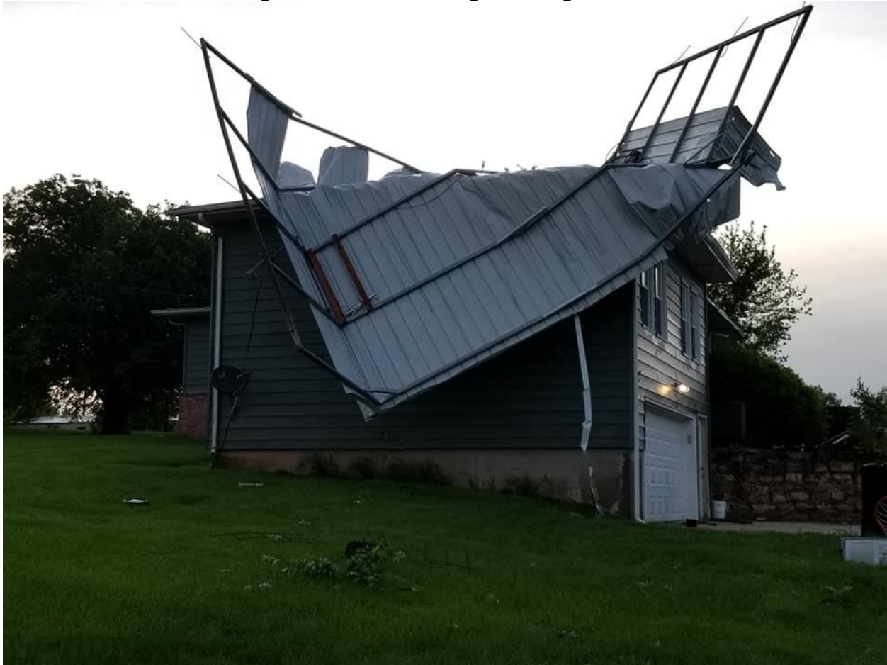
Figure STL.6: Roof Damage from High Winds
