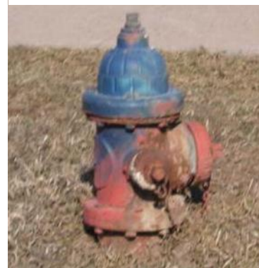
Figure 54: Inoperable Fire Hydrant in Lame Deer
