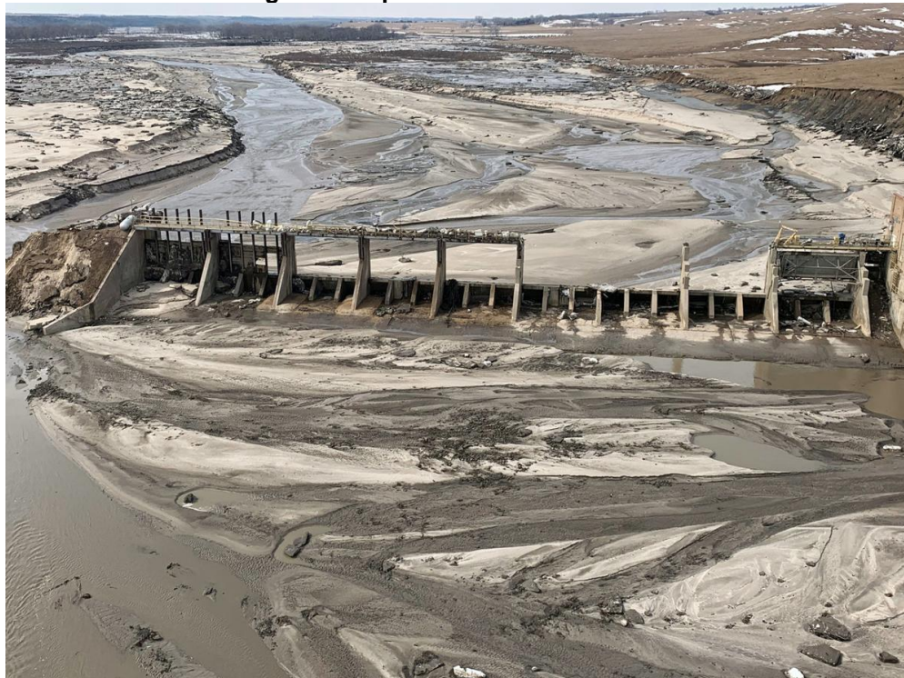
Figure 33: Spencer Dam After Breach
