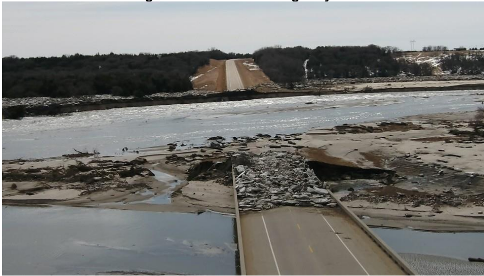
Figure 32: Washed Out Highway 281
