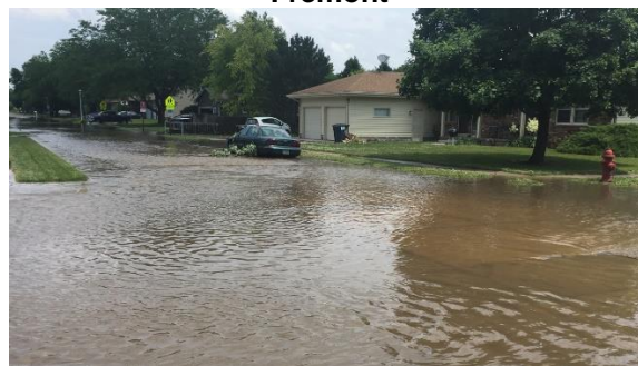
Figure DGE.7: 2016 Flooding, City of Fremont
